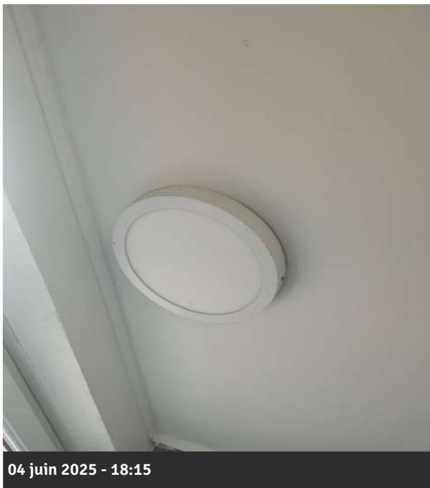
Photo 26 • Cuisine / Point lumineux
