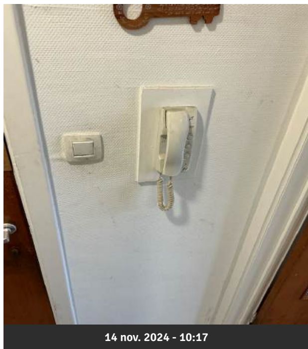
Photo 49 • Hall / Mur / Nettoyage incomplet
